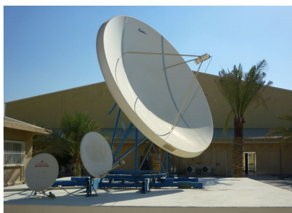
GEOLUT installed at the UAE Ground Station (AEMCC)
