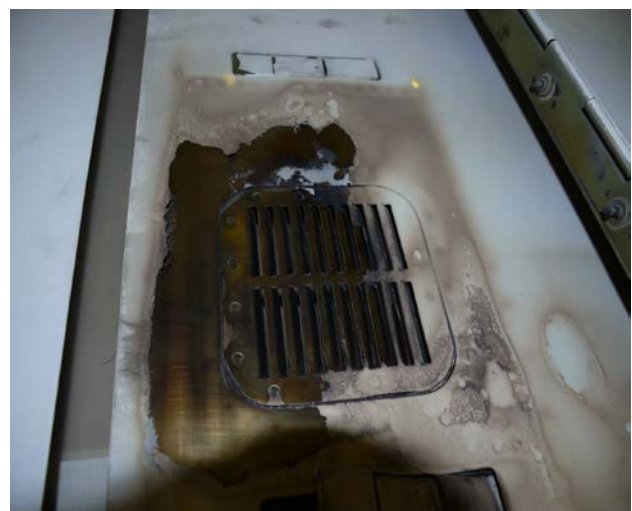
FIG 7 Close up view of 425AL with paint peeled off due to overheat
