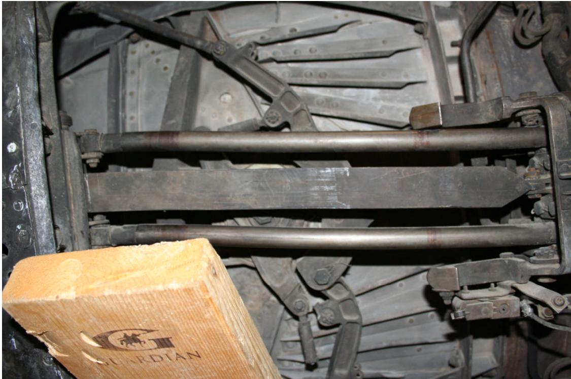
Photo (13) – Lower Actuator Rods
