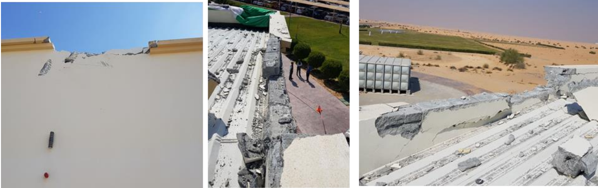
Figure 3. Damage to the building
